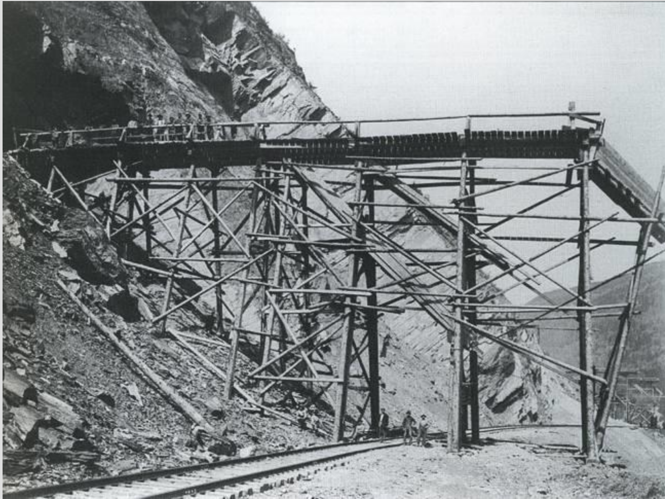
Construction on the cliff directly above the operational GTPR west of Red Pass
